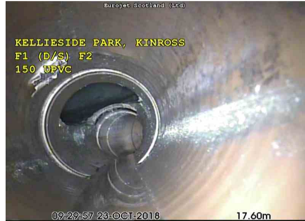
, 00:01:31, 17.60 m Broken pipe from 10 o'clock to 11 o'clock
