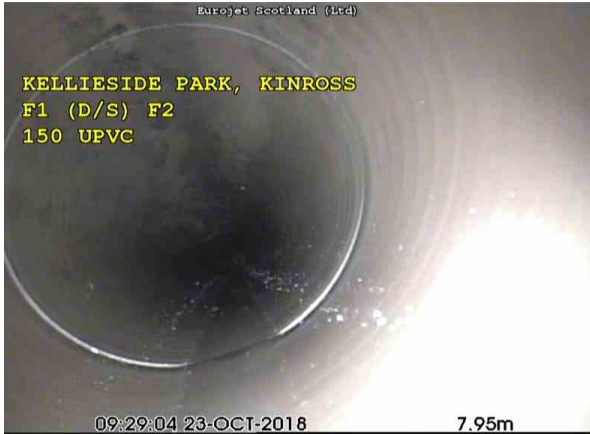
, 00:00:36, 7.92 m Deformed drain or sewer, 5%
